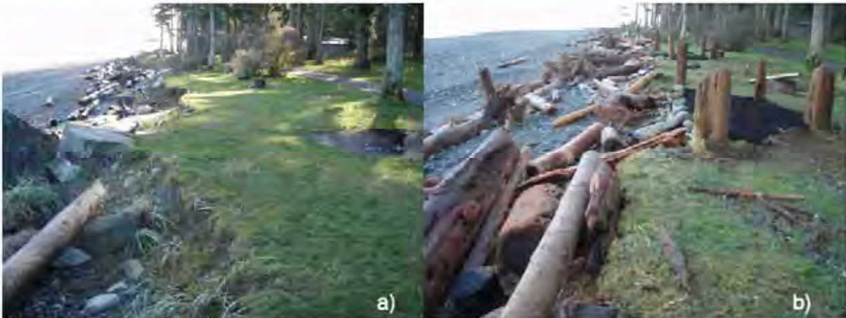
Figure 14. Views looking south along the shoreline at Kitty Coleman Provincial Park, a) prior to restoration work, and b) after the year-one project completion.
