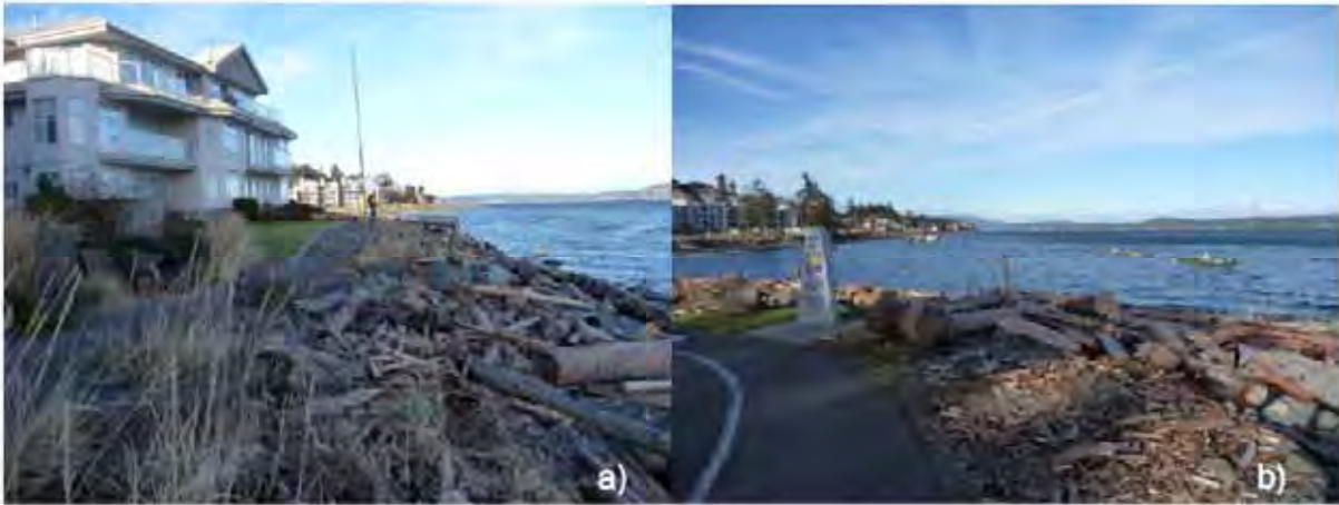
Figure A-19. Photos showing debris from recent wave runup (photos taken 17 January 2011).
